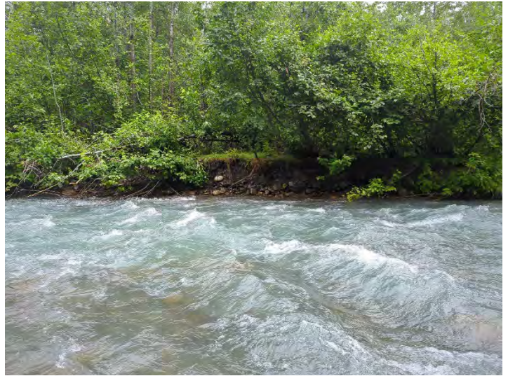
View looking across Peters Creek showing eroded drop off.
