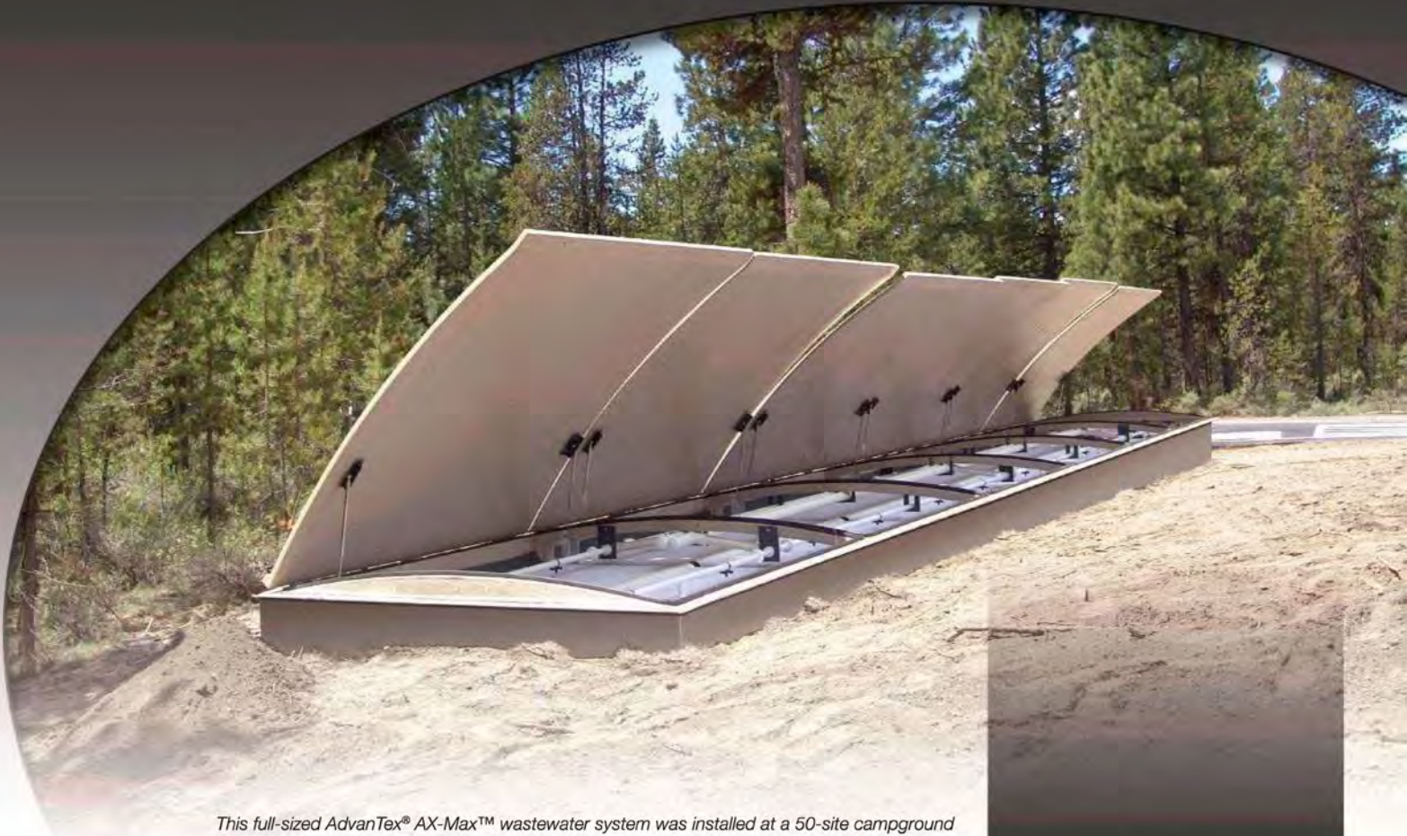
This full-sized AdvanTex ® AX-Max ™ wastewater system was installed at a 50-site campground in the LaPine State Park, LaPine, Oregon, to handle design flows of 7,500 gpd (28.4 m 3 /day).
